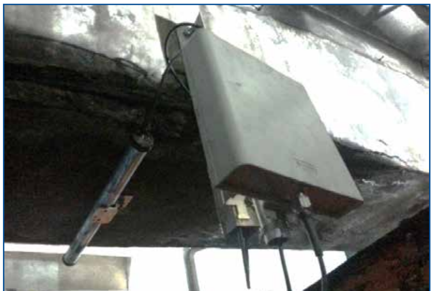
Mounted BAT antennas facilitate the wireless communication across the site.
