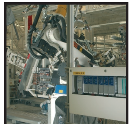
The distributors are built directly into the production cells.
